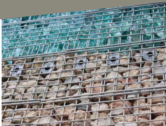
Bird boxes built into the bridge abutments – an example of habitat provided by the built environment. Monitoring has revealed that birds are using the boxes to nest and rear their young.
